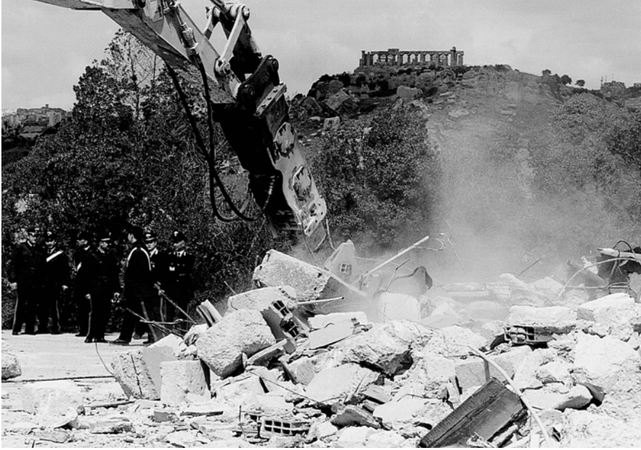
8.13 Demolition of buildings erected without licenses in the Valle dei Templi, Agrigento, March 2000
